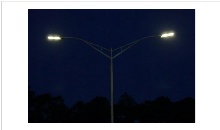
LED Traffic Lighting
