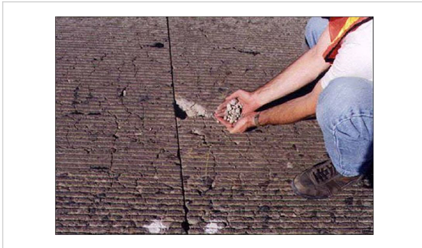
ASR Deteriorations in Pavements
